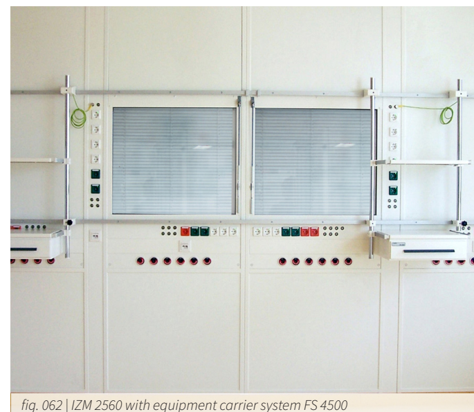
fig. 062 | IZM 2560 with equipment carrier system FS 4500
